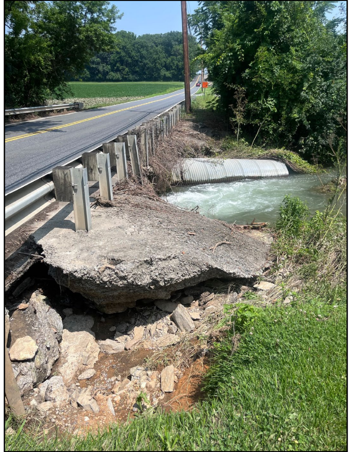
Scouring at the southeastern corner of the culvert has started to undermine Van Buren Road. A corrugated metal liner from the northern culvert was also displaced by the flooding.
