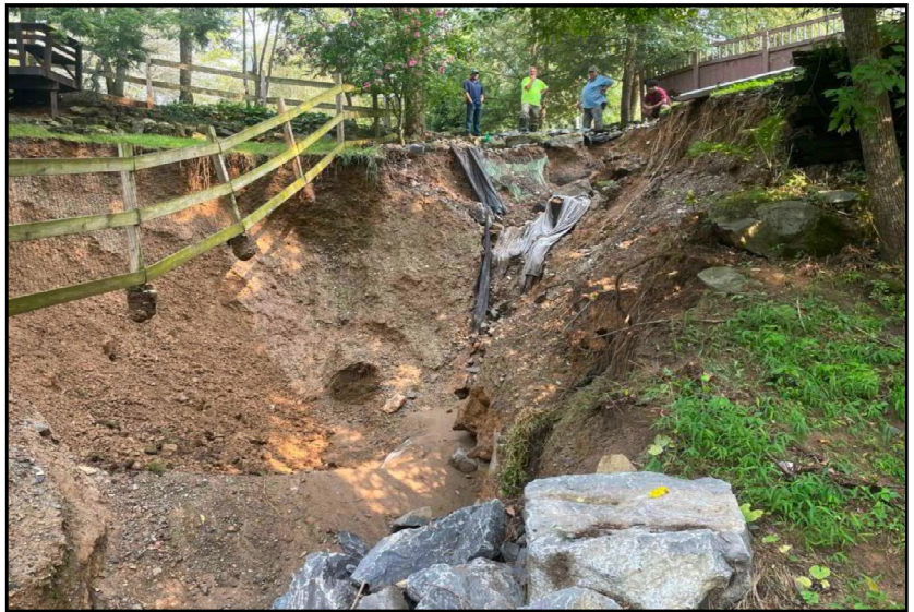
View looking northwest at a portion of the damage which occurred when a 48" stormwater sewer pipe failed during flash flooding.
