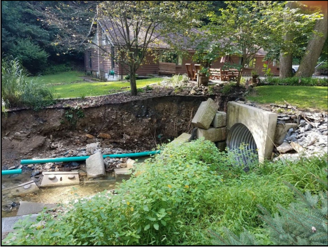
Damage to a property on Dark Hollow Road from Kreutz Creek flooding in 2018. The property was restored with the assistance of the EWP and Hellam Township
