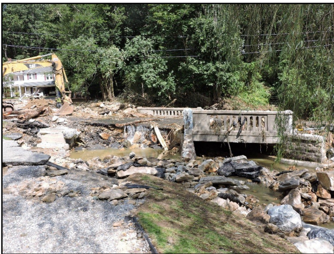
Damage to a property on Kreutz Creek Road from Kreutz Creek flooding in 2018. The property was restored with the assistance of the EWP and Hellam Township
