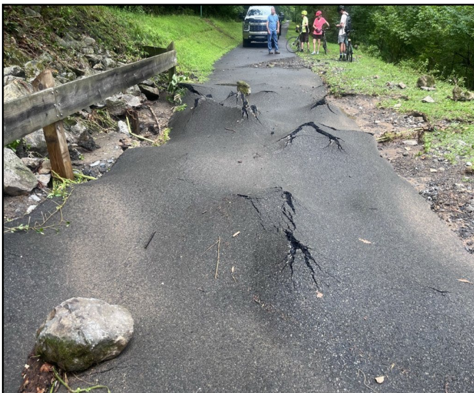
The flash flood lifted the asphalt trail surface and washed 20" rocks under the asphalt.
