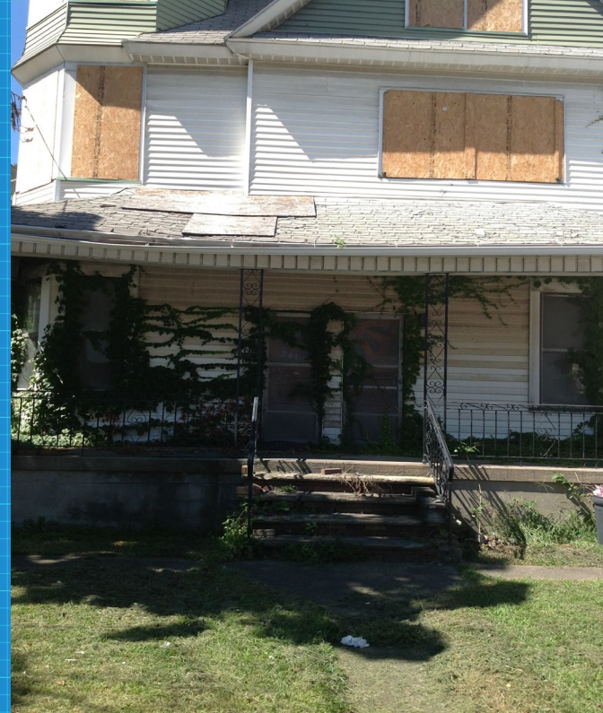
CONDEMNED DOUBLE-BLOCK HOUSE
